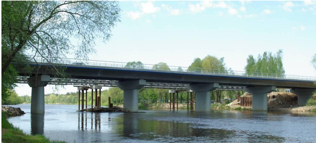
Fig.1 Strengthened piers and a new twin rib deck over the Gauja river near Murjani
