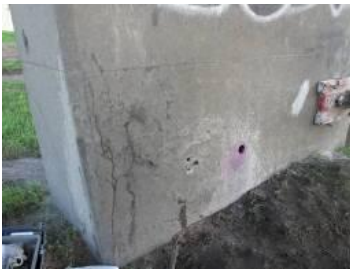
Fig. 4. Reinforcement corrosion cracks at the pier corner.
