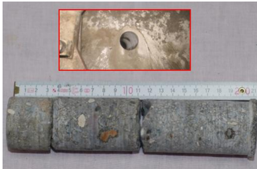
Fig. 8. Core sample from the web of the beam near leaking expansion joint
