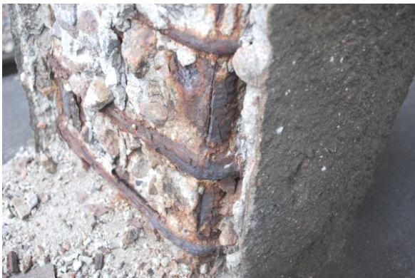
Fig. 10. Corrosion of reinforcement.
