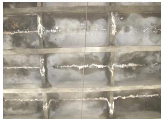
Fig. 11. Signs of leaking and deteriorated membrane.
