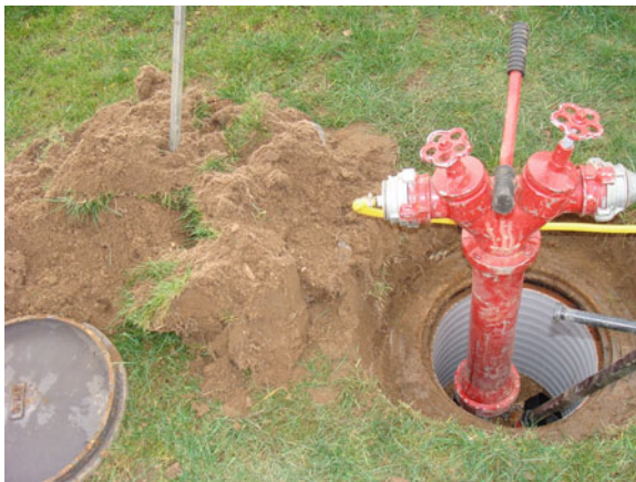
Fig. 15.14 By third person buried hydrants with clay cover
