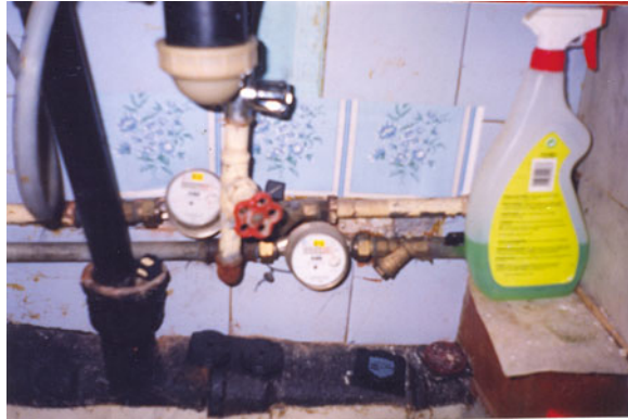
Fig. 15.2 Typical solution for installation of water meter with rotated clock face in internal piping
