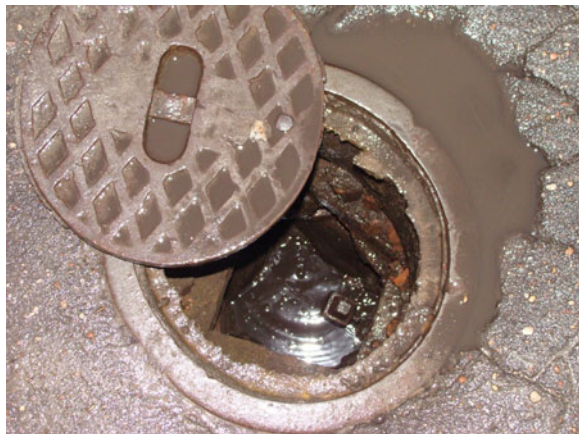
Fig. 15.12 Flooded and filled with sand Riga type hydrant (2 m in deep) due to raised groundwater level
