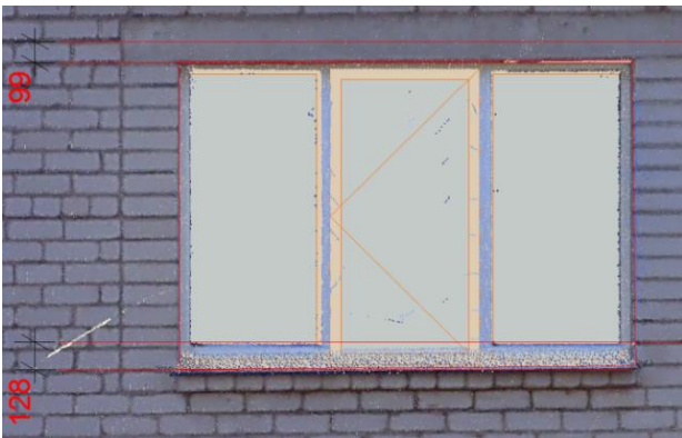
Figure 8: The height difference between left and the most right window on the North façade (red line is zero reference on 10 m base line).
