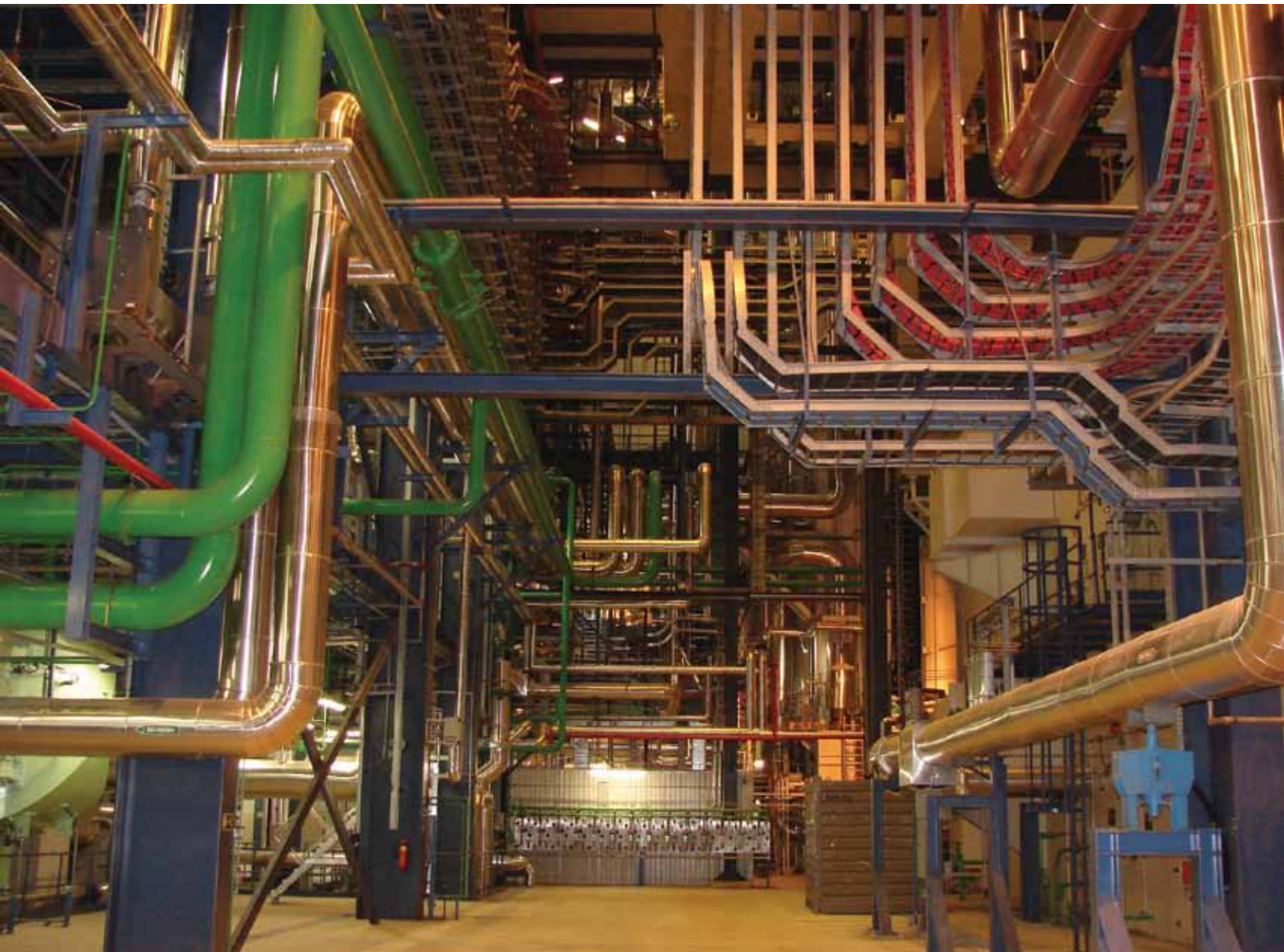
Riga TEC- 2 is the biggest newly built industrial object in the history of reinstated Latvia. Photo JSC Latvenergo.
